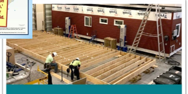
A Solar Village home being produced in the manufacturing facility in Geneva. The Solar Village company currently employs 22 people; more jobs are expected as the company builds more homes for the proposed Ithaca Solar Village.
